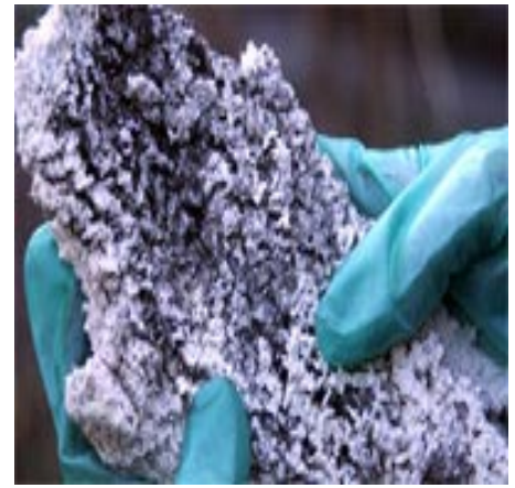
Black mold in ceiling material.
